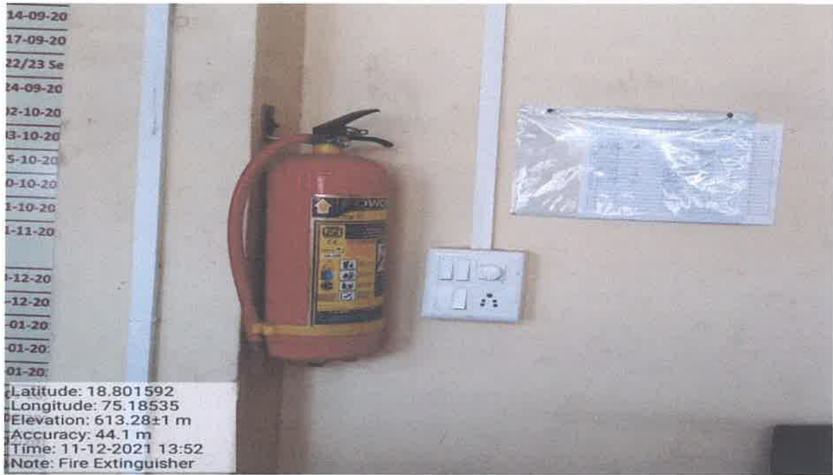
Fire Extinguisher System of Office
